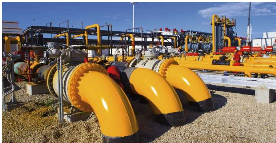
Fig. 96: Typical application field: gas compression station
