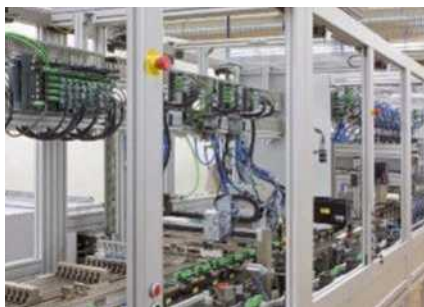
Remote maintenance: Global, direct access to controllers and Ethernet networks
