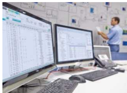
Remote control: Secure and continuous transmission of process data to the control center
