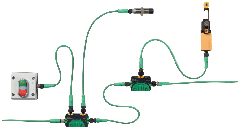
Figure 11: I/O modules with an IP67 degree of protection with SWD line to SWD modules.
