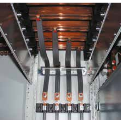
Connection: Busbar to busbar
