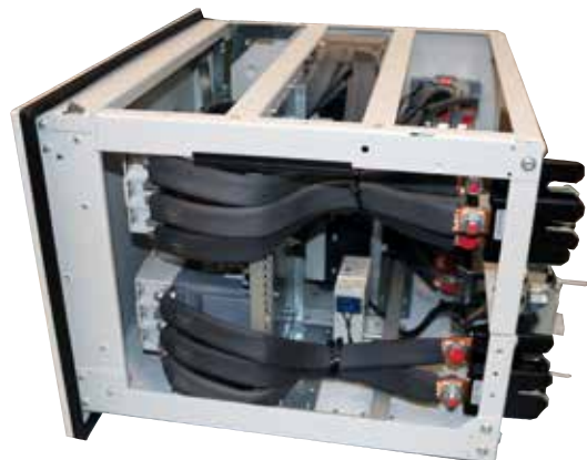
Connection: Between electrical components.
